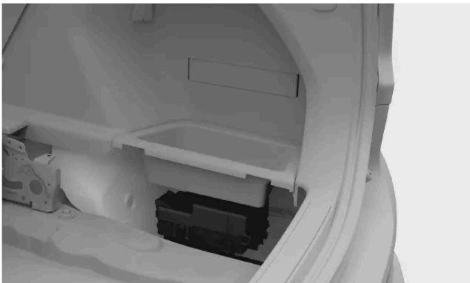
Fuse box location
