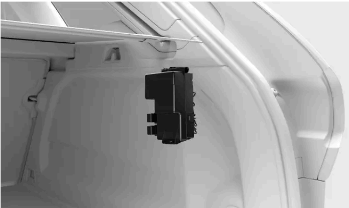
Fuse box location
