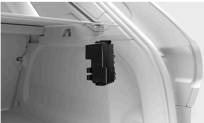
Fuse box location
